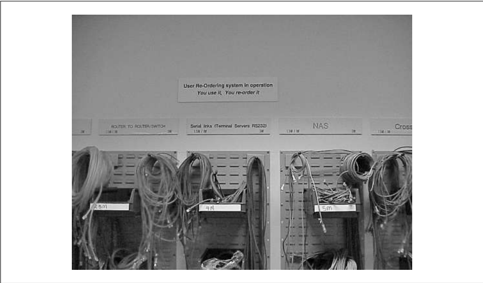
Figure 26.7: Blue bins and hanging cables at Eircom
