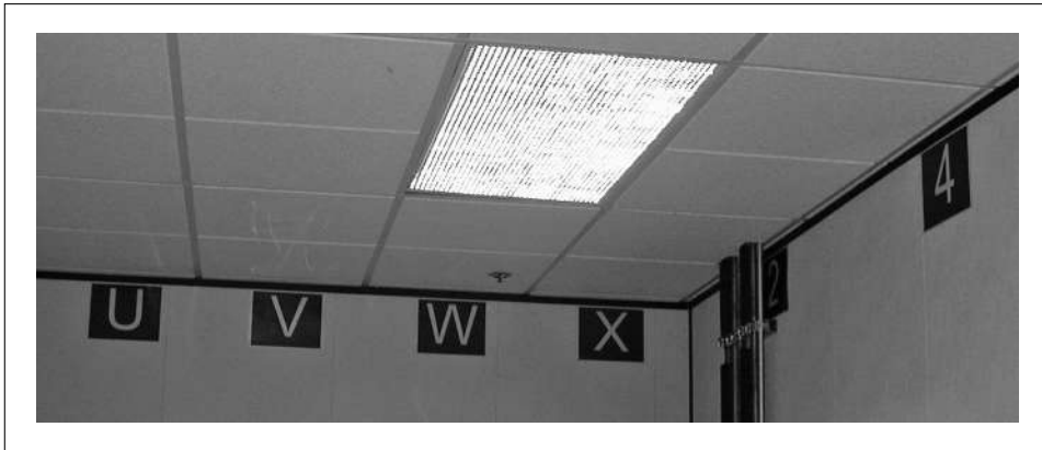
Figure 26.2: Rack numbering high on the walls at Synopsys
