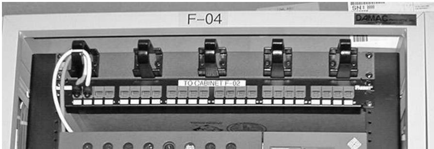
Figure 6.9 Racks at Synopsys are clearly labeled at the top and have a patch panel that indicates the rack to which it is wired.
