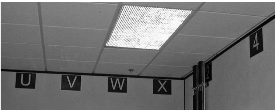
Figure 6.8 Numbering high on the walls of the data center in Synopsis is used for rack naming and makes it easy to locate a given rack.
