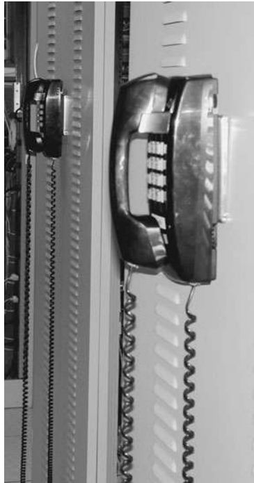
Figure 6.14 SAs at Synopsys all have radios but find that phone extensions at the end of each row work better in the data center. (Note the extremely long cord.)
