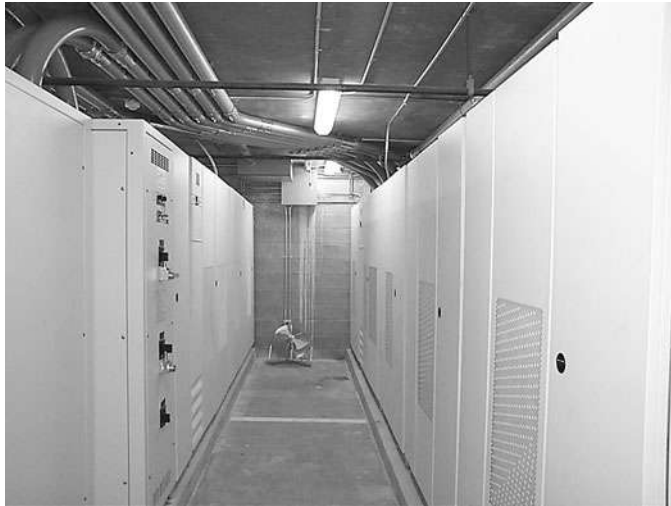
Figure 6.1 A modular UPS at GNAC, Inc.
